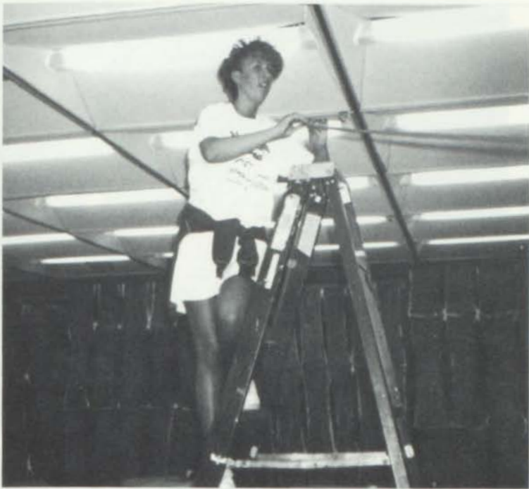
COMPLETING the top of the bamboo hut is junior Heather Johnson. The eating area was built as one large bamboo hut. —S. Hatcher
